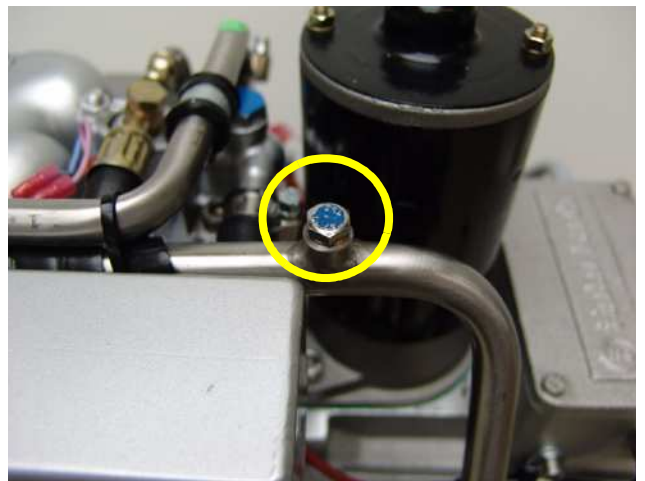
Fig. A.3.3-6: Ventilation screw cooling water pump
