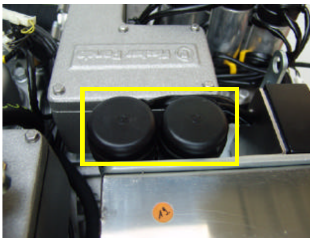
Fig. A.48: Booster capacitors
